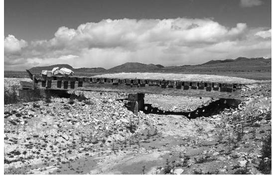
A view of what was once a cantilevered trestle, separated from the railroad grade on both ends and balanced on the central pier only. The BLM has now stabilized this trestle. Photo by Ray Kelsey.
