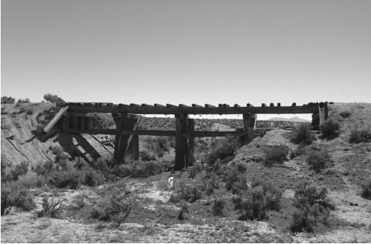
A trestle near Lucin, Utah, that has been heavily undermined by seasonal flooding, exposing the bases of the piers. Photo by Ray Kelsey.
