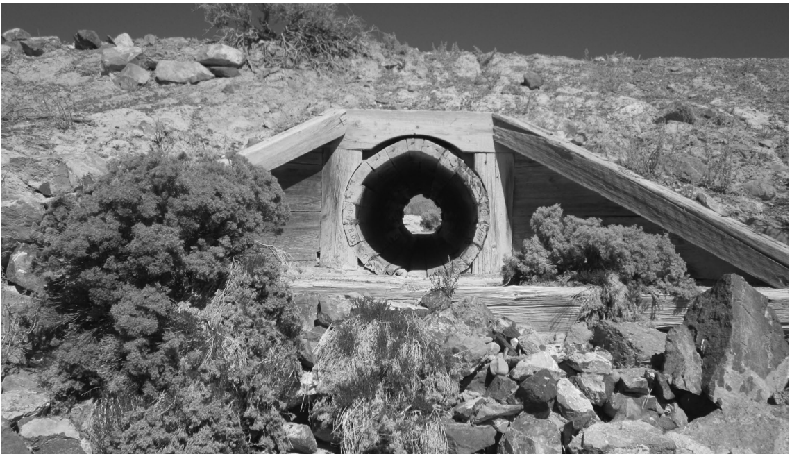
A wooden culvert, likely constructed in the 1870s–1880s. Photo by Glenn Stelter.
